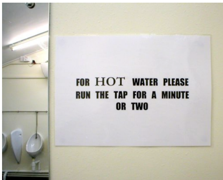
Figure 11. Energy and water wastage due to dead legs is a daily experience.
