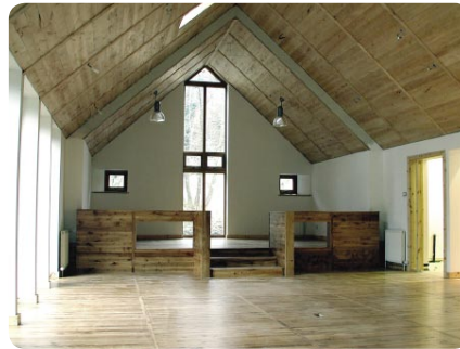
Glencoe Floor - the flooring at the Glencoe Visitor Centre is nail-free - designed for easy removal, replacement or reuse by being loose laid and held at the ends by screwed battens. (Gaia)
