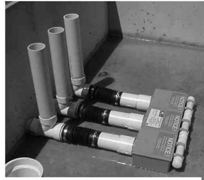
Figure 3. Three units joined and extended for increased draw-down and even dosing to three trenches of a large leachfield system.
